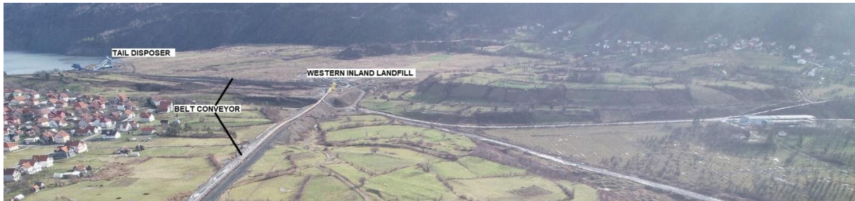
Figure 4 Current state of works in the area of the former Čubrić mine
