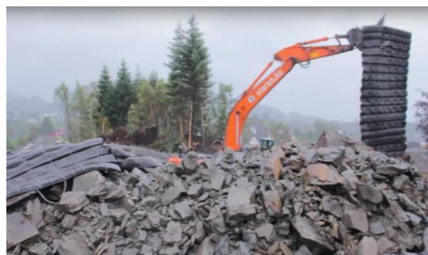
Figure 3 Removal of blasting mats after blasting from a muck pile with a hydraulic excavator [13]
