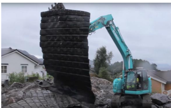
Figure 2 Placement of blasting mats on the blast field during blasting in urban areas [13]
